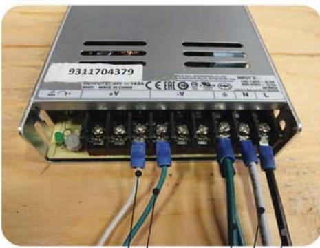
To Power Harness + (White) - (Green) 24 V going out Earth Ground (Green/Green) Neutral (White) Hot (Black) Connected to 120 AC Power and 220 AC Power
